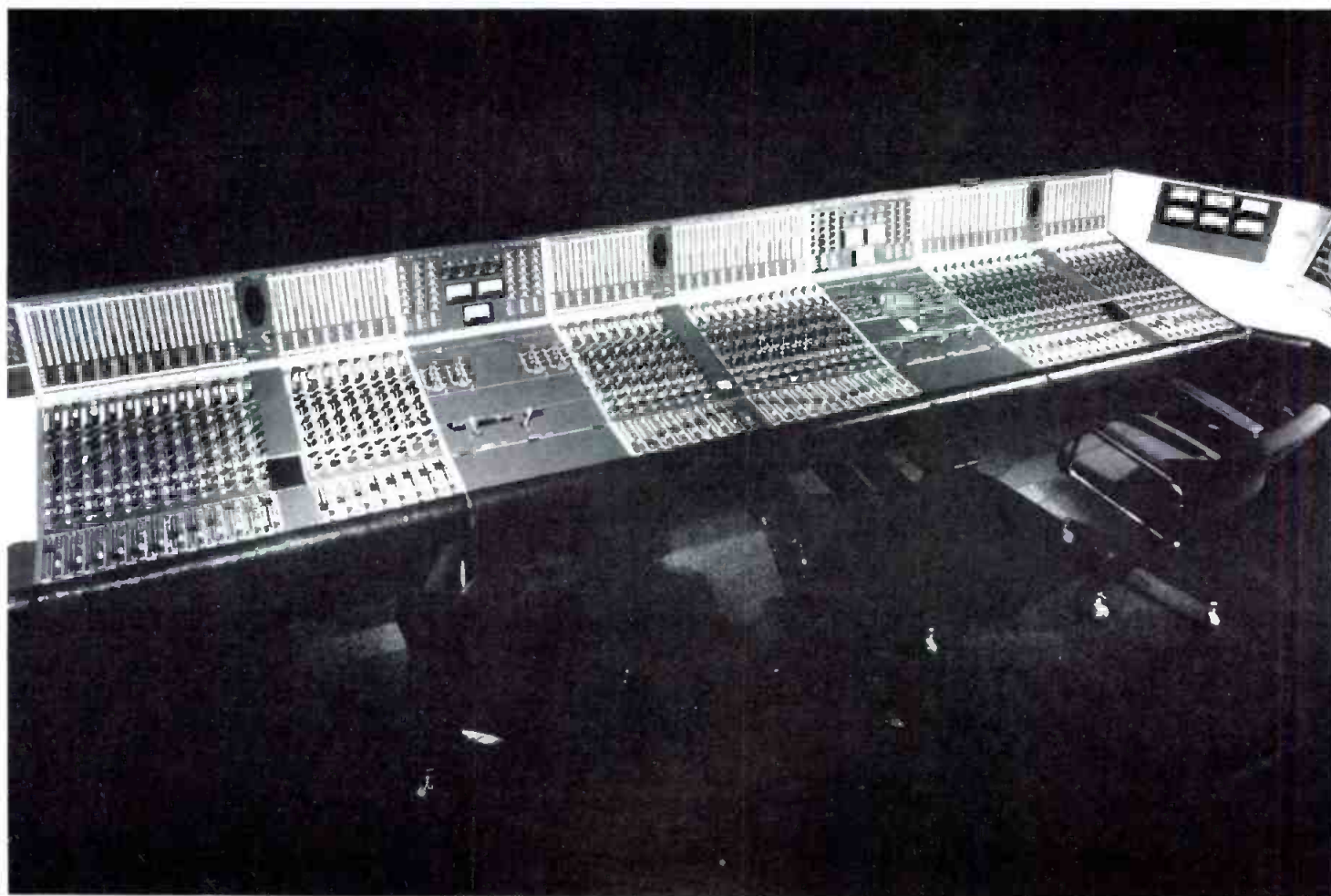
Figure 1. The new console in Pinewood's Theatre 2.
